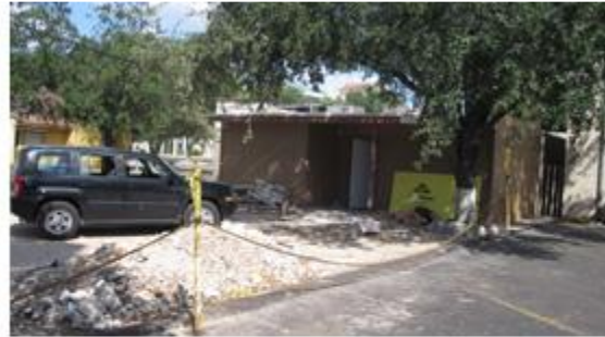
This is the rear entrance to Whole Women's Health, an abortion clinic in McAllen, TX. It is in a gross state of disrepair. Many of the violations discovered during a three month investigation were from this clinic.
