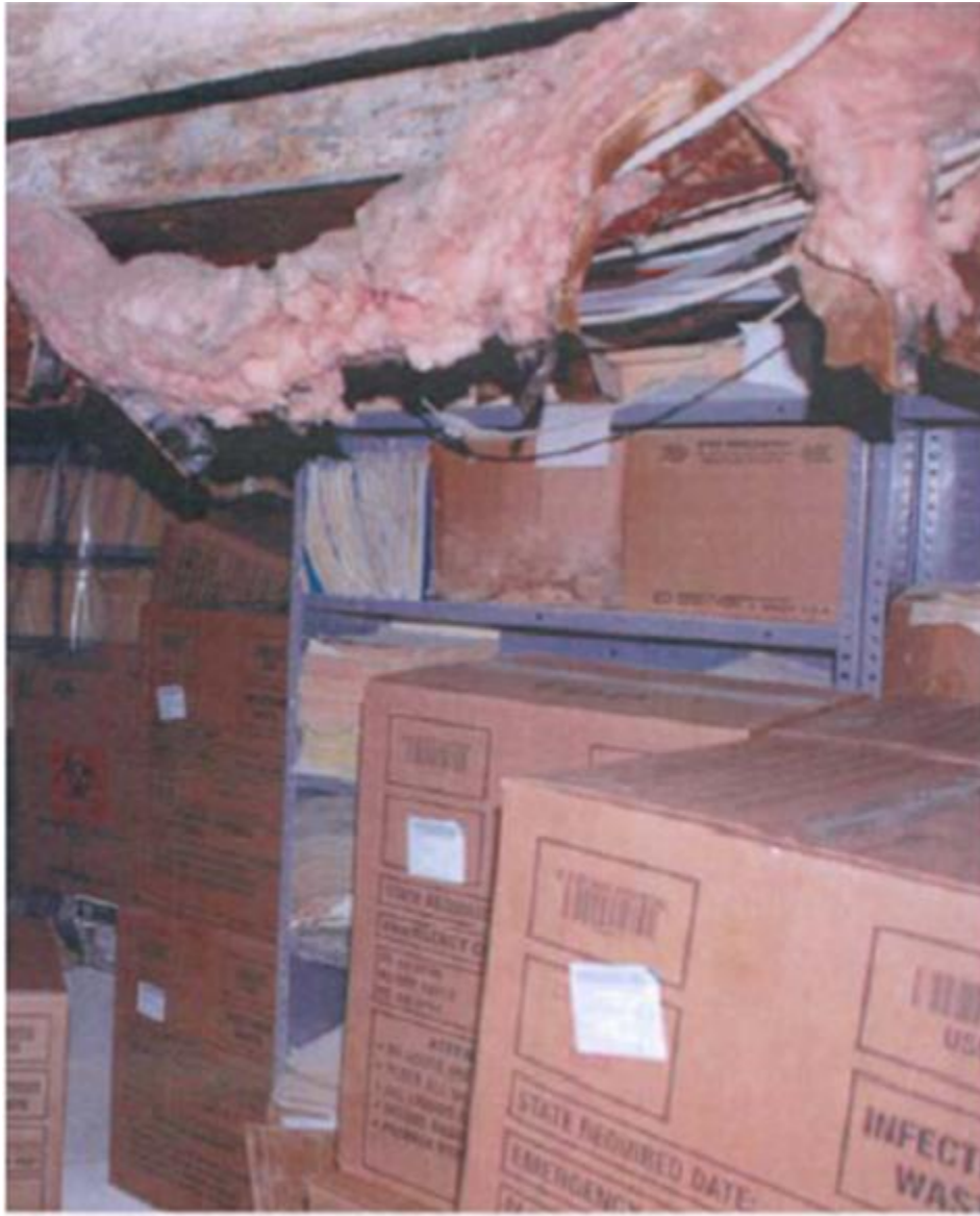
Boxes of bio-hazardous waste in basement
