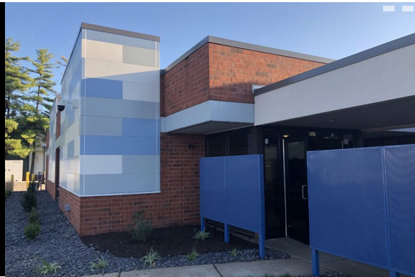
The exterior of a new Planned Parenthood facility that is under construction in Fairview Heights, shown in an Oct. 2, 2019, photo. Photo by Kim Bell.
